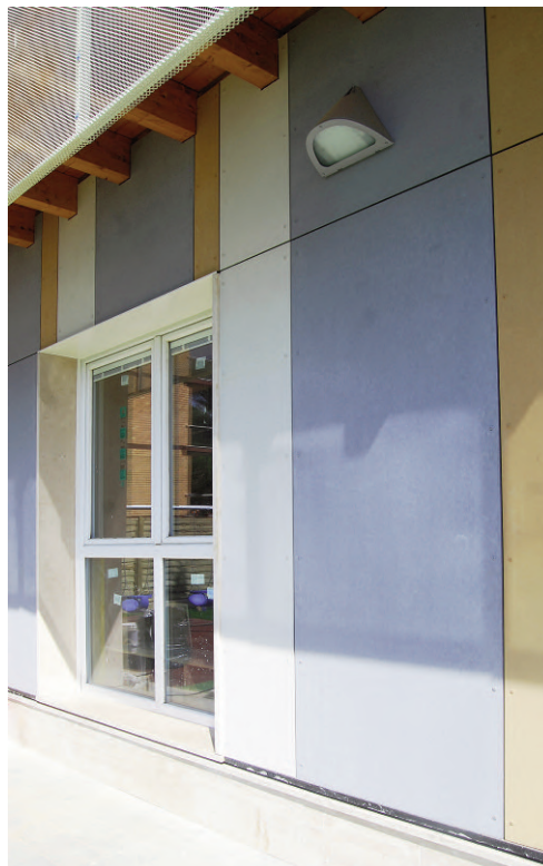
Figgs. 12, 13 - Details: The substructure of the ventilated façade in fiber-cement slabs, made with wood slats; The façade covered in dry-mounted fiber-cement slabs, with the effect of solar shading given by the metal mesh panels (credits: P. Altamura, 2017).
