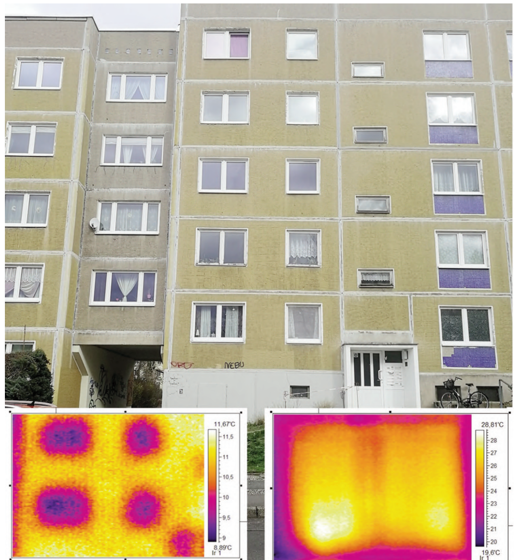
Fig. 10 - The district of Loßnig, Block in Gersterstrasse 12-24: thermal analysis with the infrared camera to the series WBS70/10800/5, Leipzig 2019 (credit: M. Block, 2019).
