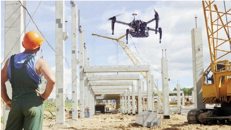
Fig. 1 - The use of drones facilitates risk analysis on site and ensures greater safety ( www.dronezine.it/40400/dagli-usa-cinque-lezioni-usare-droni-nelledilizia/ ).
