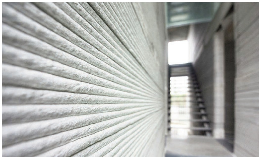
Fig. 10 - Concrete box, prints layer by layer with the typical texture (photo by WinSun).
