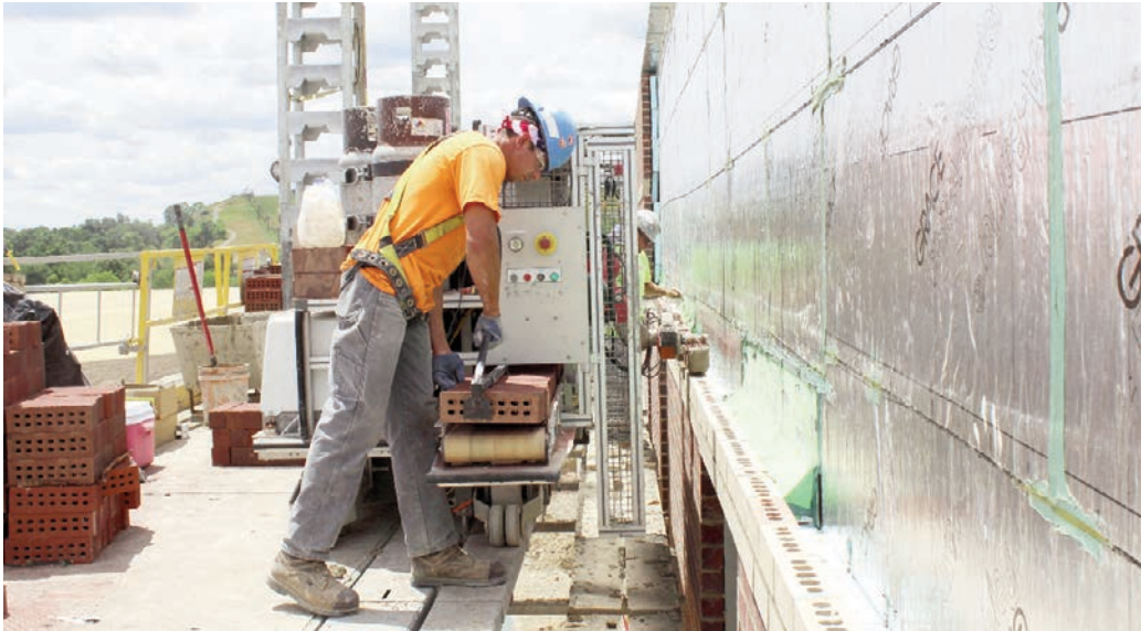
Fig. 7 - SAM/100 bricklaying robot, masons work together at the University of Michigan Brighton hospital (photo by Construction Robotics).
