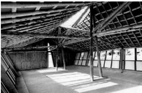
Fig. 10 | The 'Big Shed' Assembly Workshop (2012) by AA Design & Make with Mitchell Taylor Workshop and Atelier One (credit: V. Bennett, 2012).
