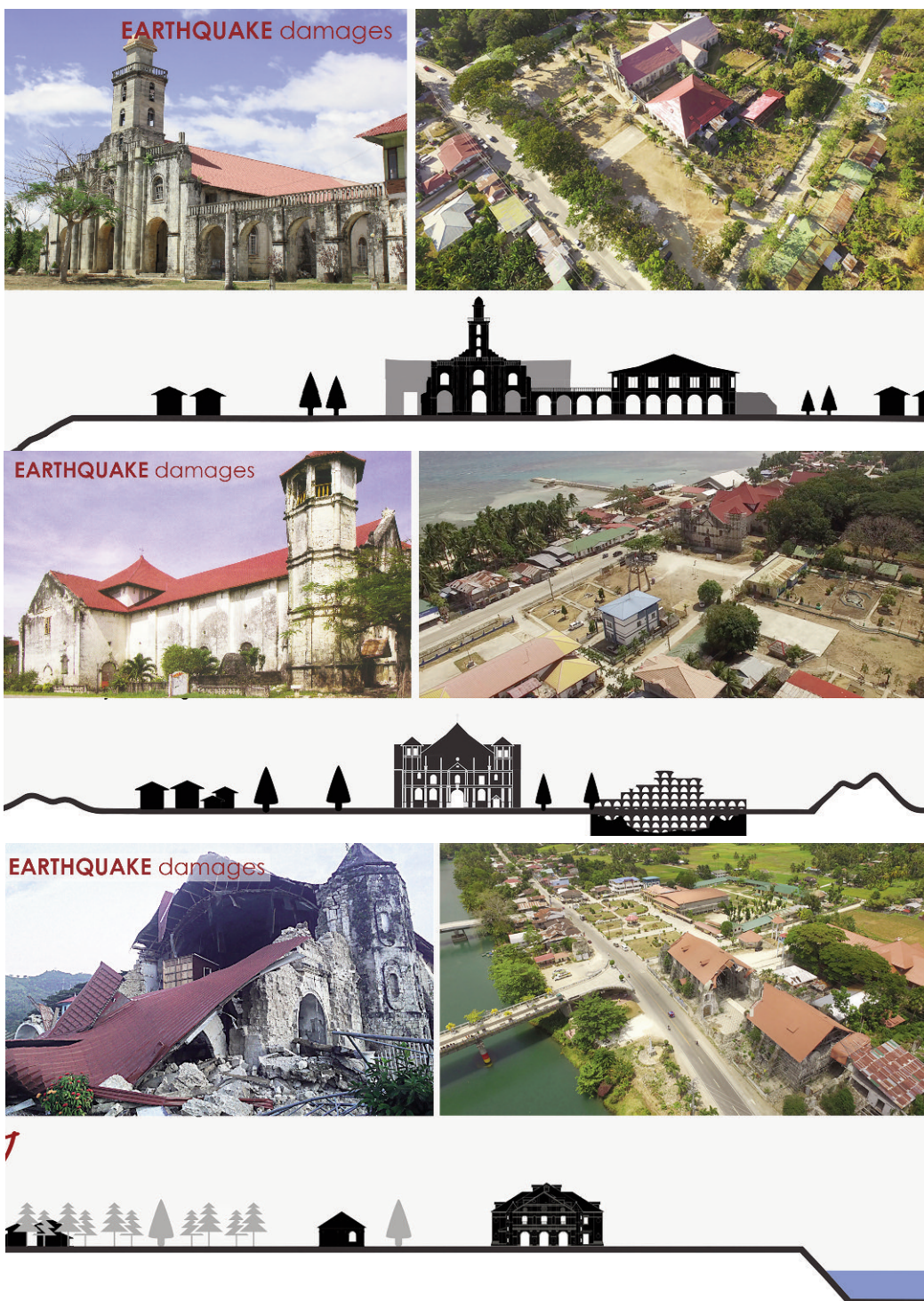
Fig. 2-4 - From the top: Post-earthquake damages in Santa Monica Church, Albuquerque, Bohol, Philippines (photos UPD's, drawings S. Schiazzano 2016); Post-earthquake damages in San Nicola Tolentino, Dimiao, Bohol, Philippines (UPD's photos, drawings F. Vardaro, 2016); Post-earthquake damages in San Pedro and Pablo, Loboc, Bohol, Philippines (UPD's photos, drawings A. Mustilli, 2016).
