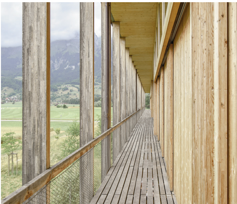
Fig. 6, 7 | Construction site photographs taken during the installation of the prefabricated façade panels (credits: Blumer Lehmann | Claude Hausammann, 2017).
