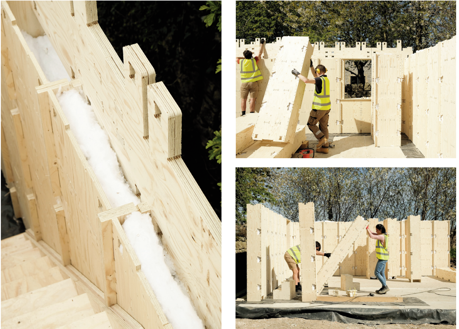
Figg. 2-4 | WikiHouse, a stage in assembling a prototype of the WikiHouse Skylark building system (credit: J. Watts, 2022).
