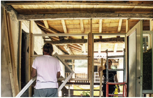
Fig. 8 | A phase of the Workshop of Thesis conducted in 2021 at Casamatta – Legambiente Varese, in Malnate (VA), AUIC School – Politecnico di Milano: the workshop envisaged the design and realisation of perimeter walls using reclaimed doors and windows and building components, identified in the area through the RE-sign platform (credit: M. Zanini, 2021).
