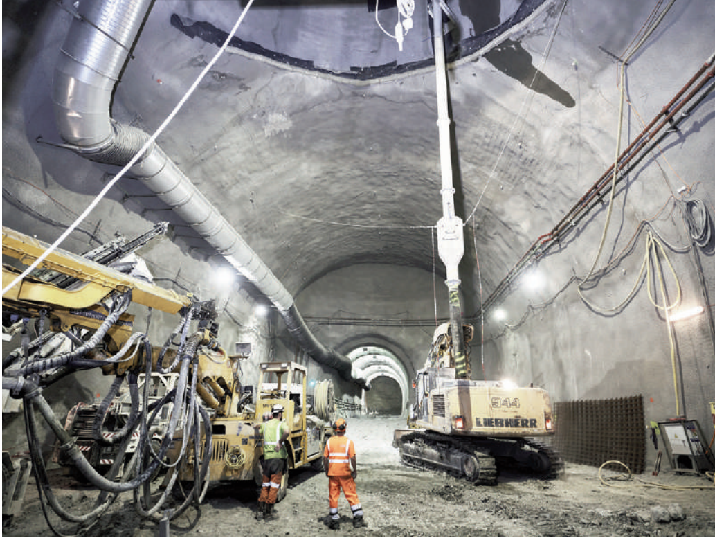
Fig. 7 | Tunnel work for the future High Luminosity Large Hadron Collider (HL-LHC), 16 August 2019 (credit: M. Brice, CERN Photos Archive).
