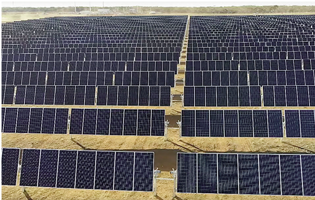
Fig. 1 | Sunraysia Solar Farm, Australia (credit: UNSW, Sydney).
