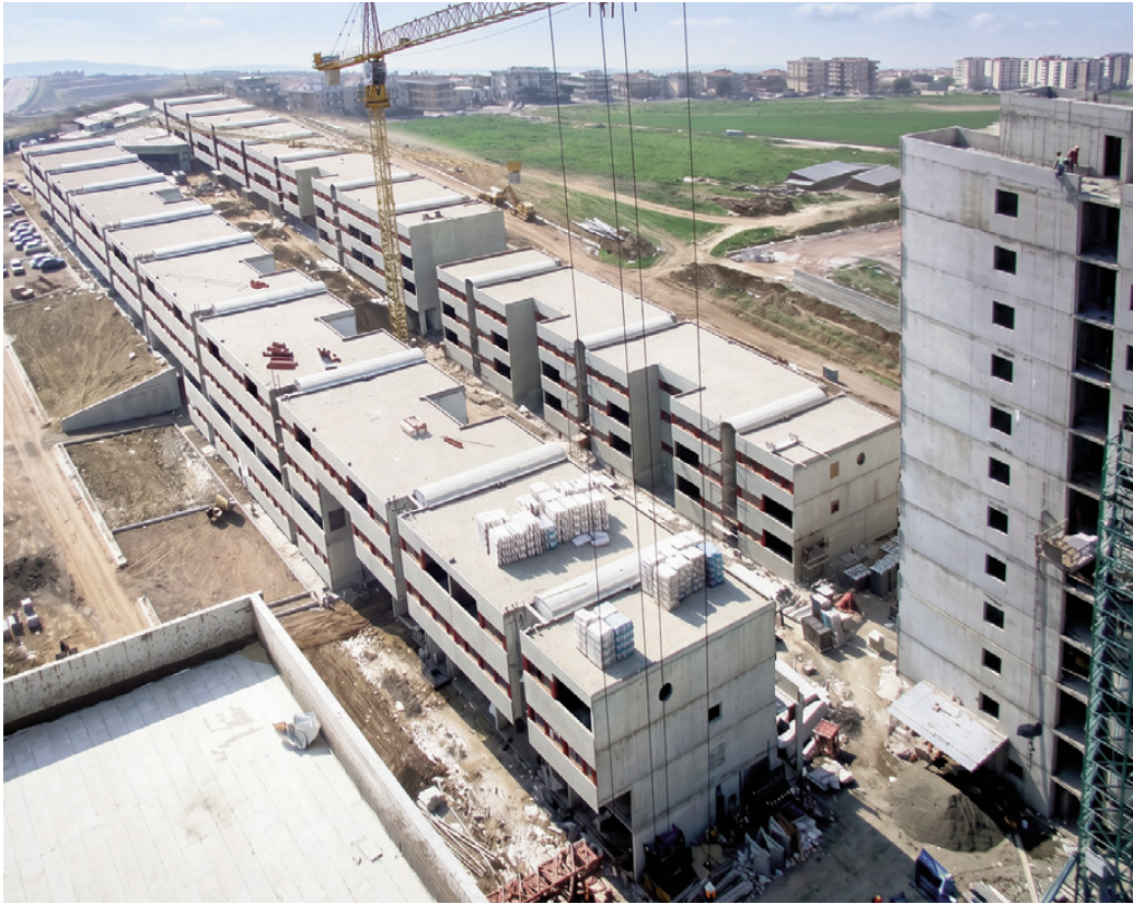
Fig. 1 | Torrevecchia (Rome, around 1980): the building site and the tunnel formwork construction system (source: Archivio Studio Passarelli).
