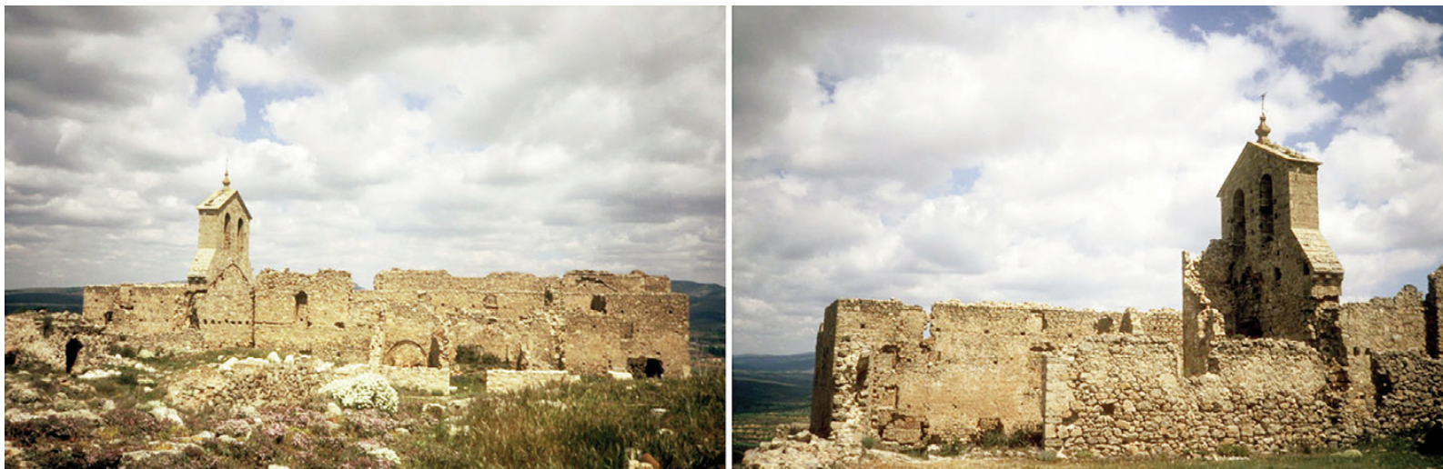
Fig. 8 | Former Church of La Trinidad in Moya prior to intervention, documenting the deteriorated condition of the historic masonry fabric and the loss of the original roofing and structural elements (credit: the Authors, 2026).
