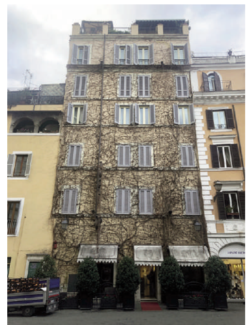
Figg. 4, 5 | Summer and Winter aspect of a vegetated building in Rome, Italy (credits: L. Herzog, 2018, 2020).
