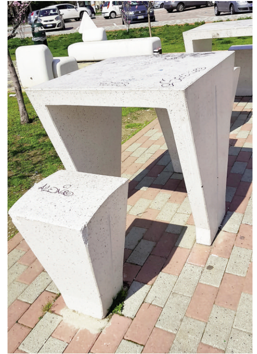
Fig. 7 - Urban furniture stools and tables made of self-compacting concrete and polished artificial stone: colour variation, local staining and graffiti (operating life: 4 years); Parco Mennea, Turin (credit: R. Maspoli, 2019).
